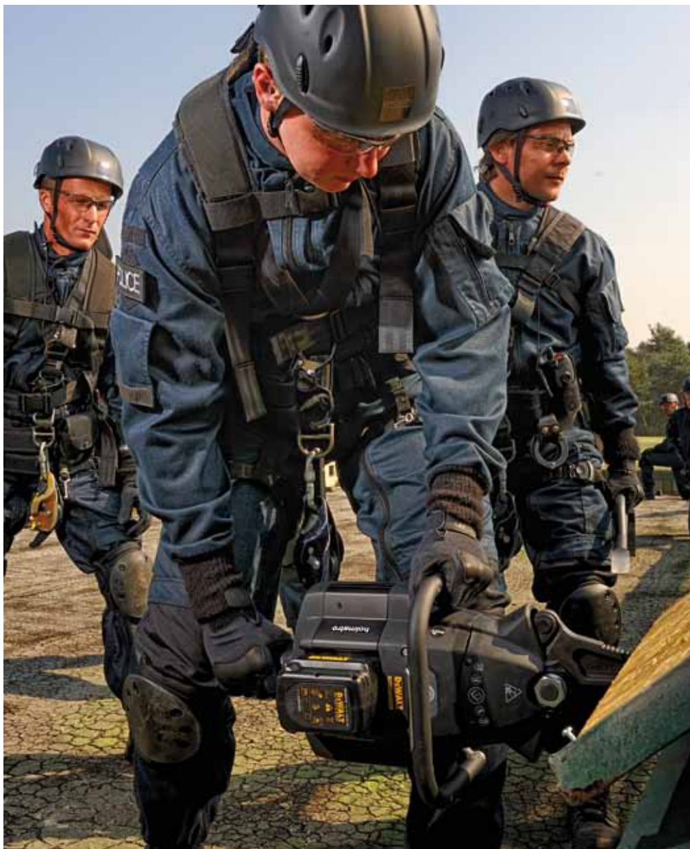
Spreading open a roof hatch and cutting the barred window (see page 8) with a Holmatro battery-operated combi tool.
